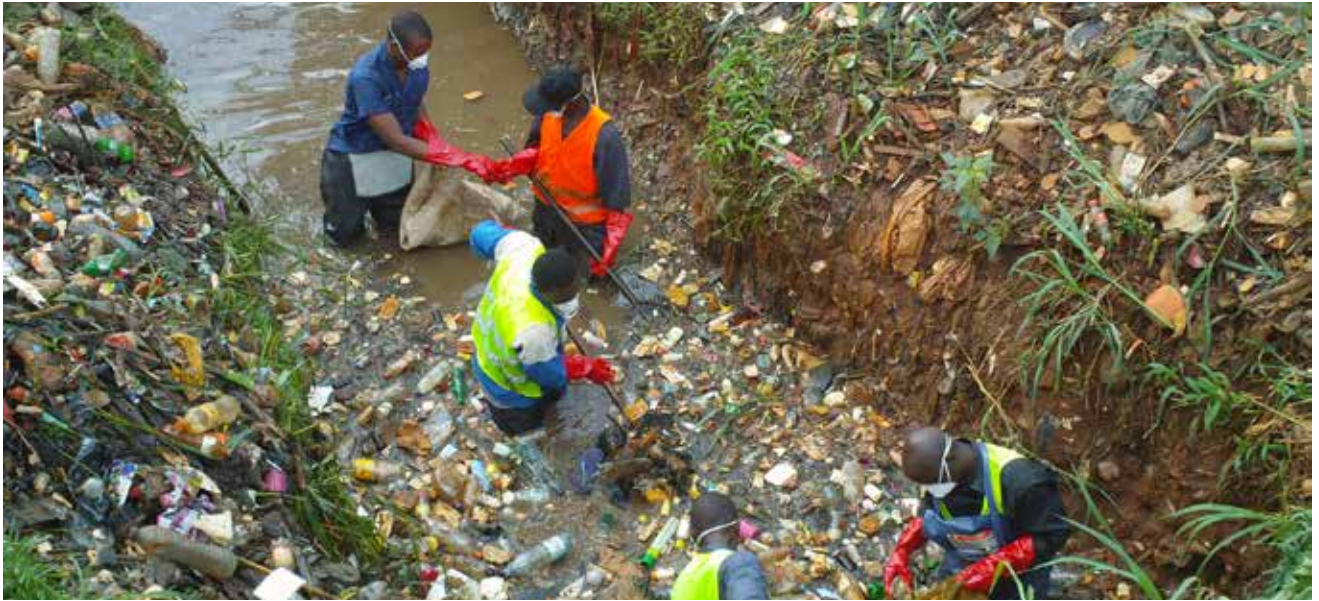
Cleaning of the Edzoa-Mballa River (AREM) as part of the community-managed fund PSUP phase 3 project in Nkol-Bikok slum, Yaoundé, Cameroon. Photo credit: PSUP country team in Cameroon.
